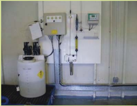
Huwa-San Peroxide Dosing system at NHS Hospital in the UK.
